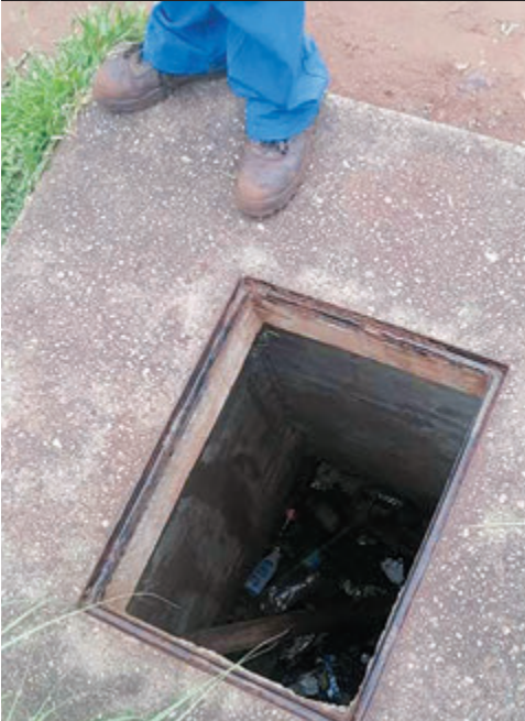
The open hole, an estimated 2 metres deep, located near Ysterberg Primary School.
